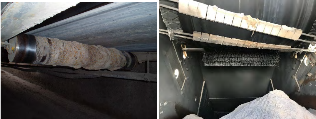
Figure 1 (left): Typical build-up of carry back on return roller from insufficient belt cleaning. Figure 2 (right): Dual primary ceramic cleaners and motorised brush secondary.
