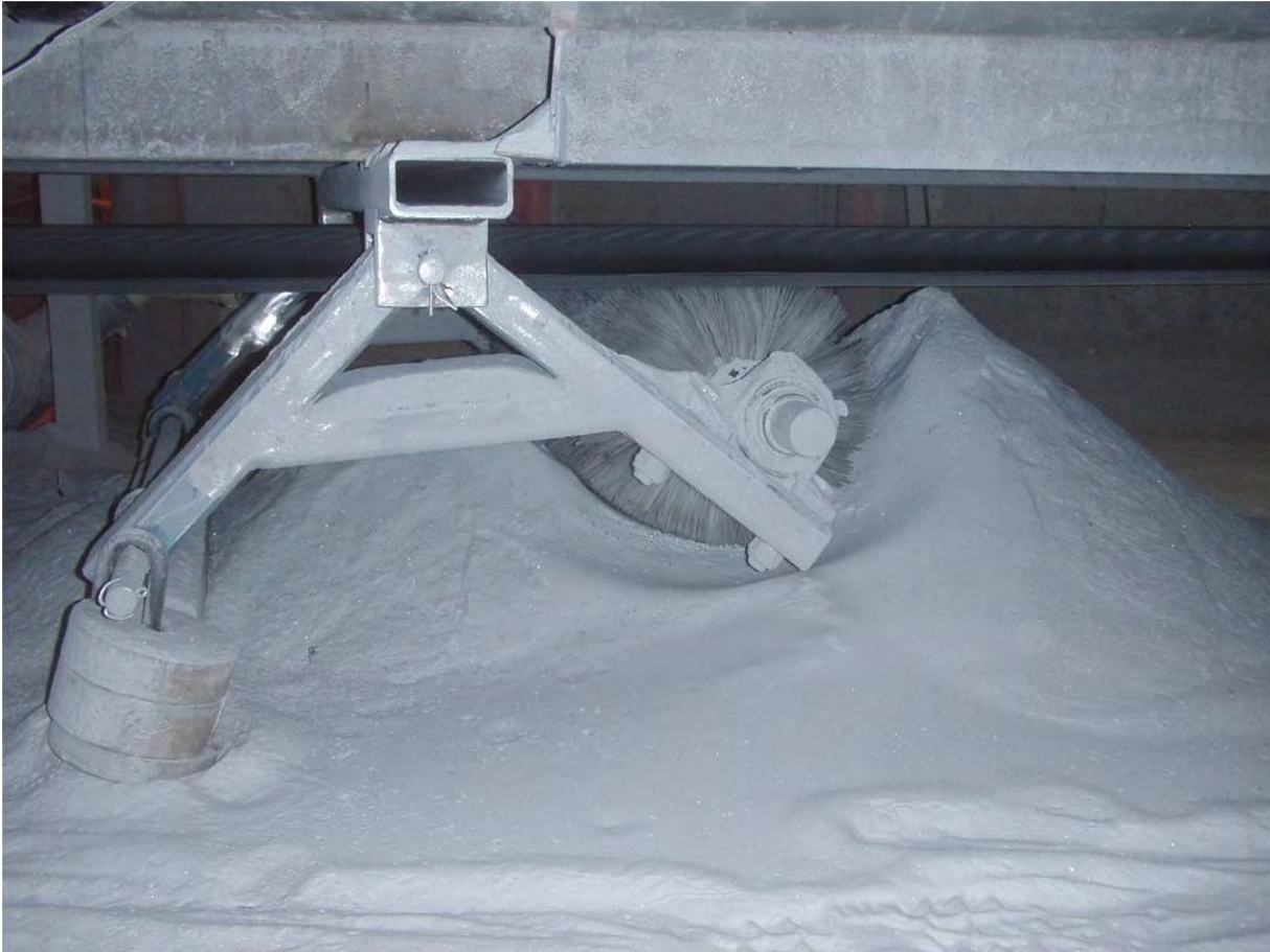
Figure 7: Non-powered brush cleaners can be installed slightly off perpendicular to the belt direction. This demonstrates the need to plan cleaner placement thoughtfully.
