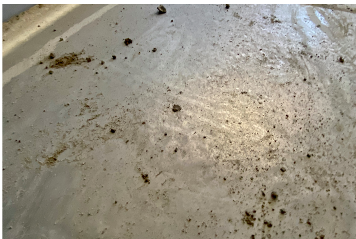
Image: K-Floshield® after install shows no signs of wear and maintains original shine and slipperiness. Hang up issues resolved.
